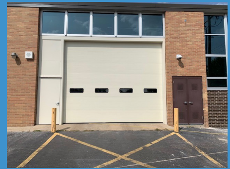
Above and Below: New garage doors, windows, inside doors and electrical service were all a part of the renovations.
